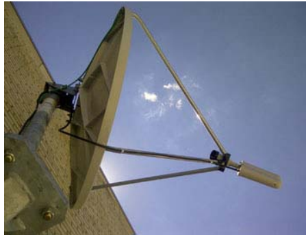
Roof mounted Satellite Dish
