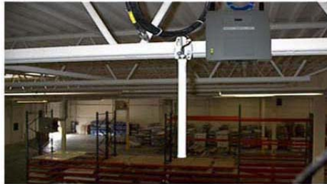
Warehouse installation of an access point
