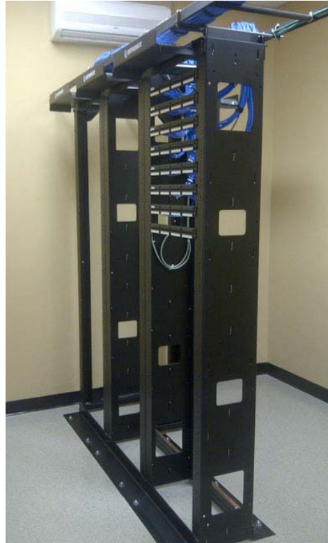
Category 6 Structured Wiring System
