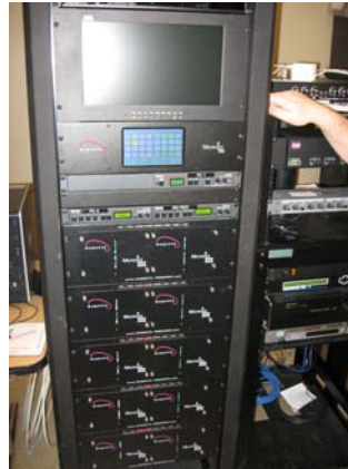
Headend Video Distribution System
