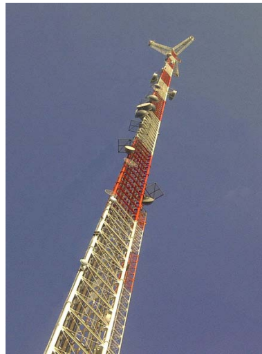
Cellular Radio Tower
