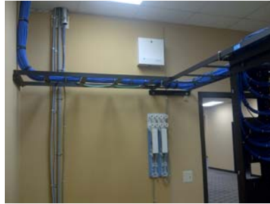
Cable Tray in Wiring Closet
